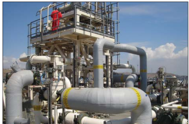
ULVA Shield offers corrosion protection to major oil & gas pipelines in Azerbaijan.
