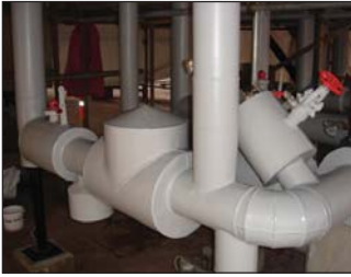
Valves protected from corrosion by ULVA Shield, Fife, Scotland.
