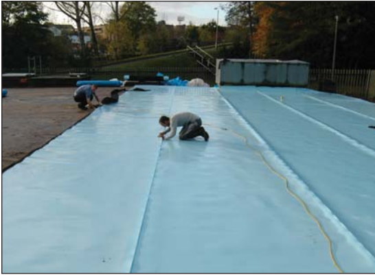
Hylam IQ installation at Wilmslow water works for United Utilities Water Authority.
